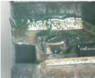
[Corrosion of contact]
